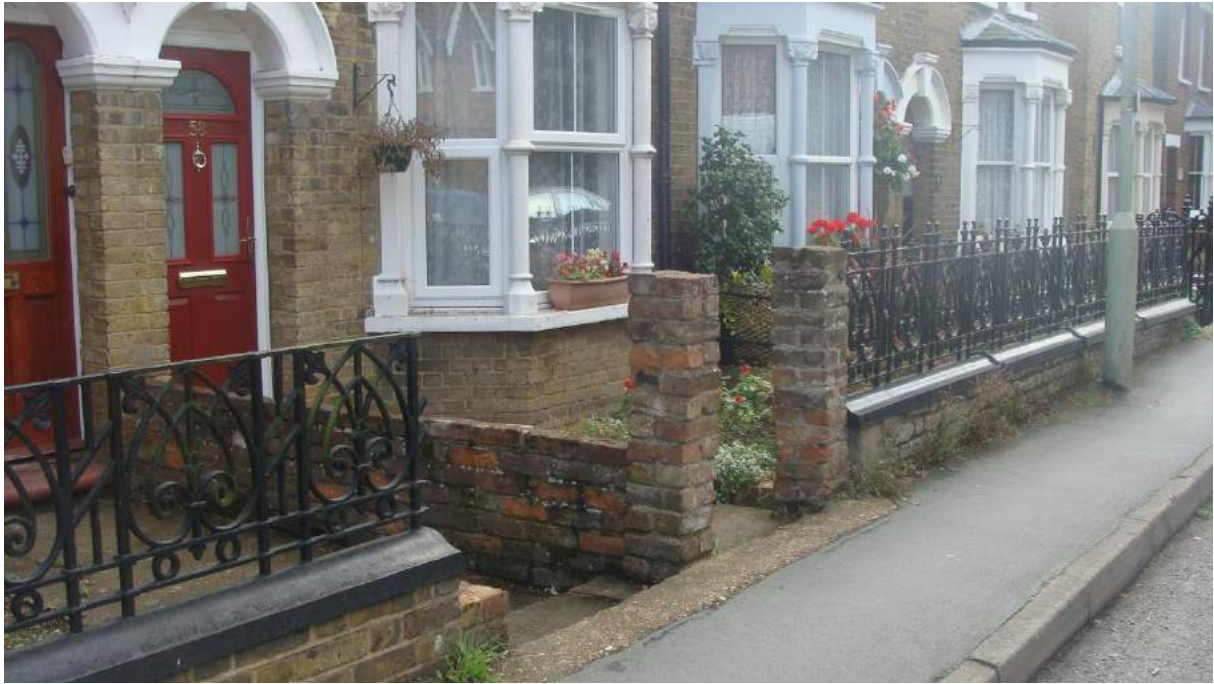
Picture 12. Good quality unlisted boundary wall and railings. Substantial demolition would require planning permission but alteration or partial demolition such as the removal of gates could only be controlled via the introduction of an Article 4 Direction restricting alteration.
